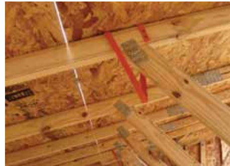
A pre-installed attic anchorage system.
